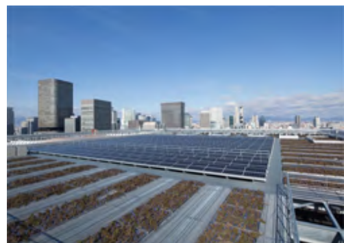
Rooftop solar panels at the Osaka Head Office (East Building)
