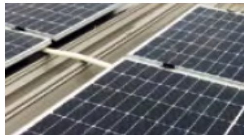
Rooftop solar panels at the Okegawa Sales Office of the Saitama Branch
